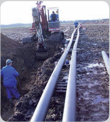
Industrial waste heat pipeline
